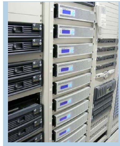
10 Cerify systems installed in the master control room
