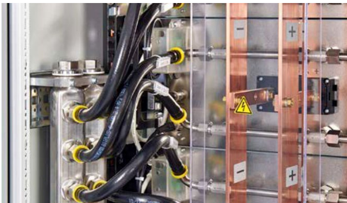
Figure 3 Close-up of the water distribution of the 240 kW cabinet with eight units and water cooling.
